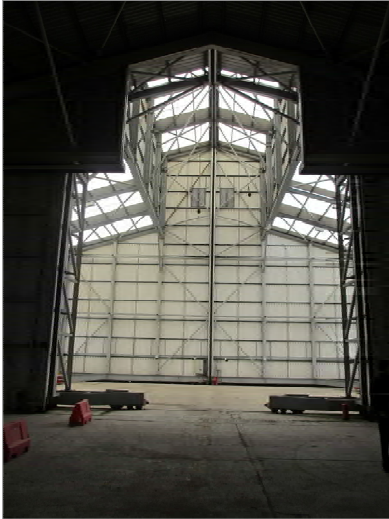
Figure 16: Bespoke tail enclosure of hangar
