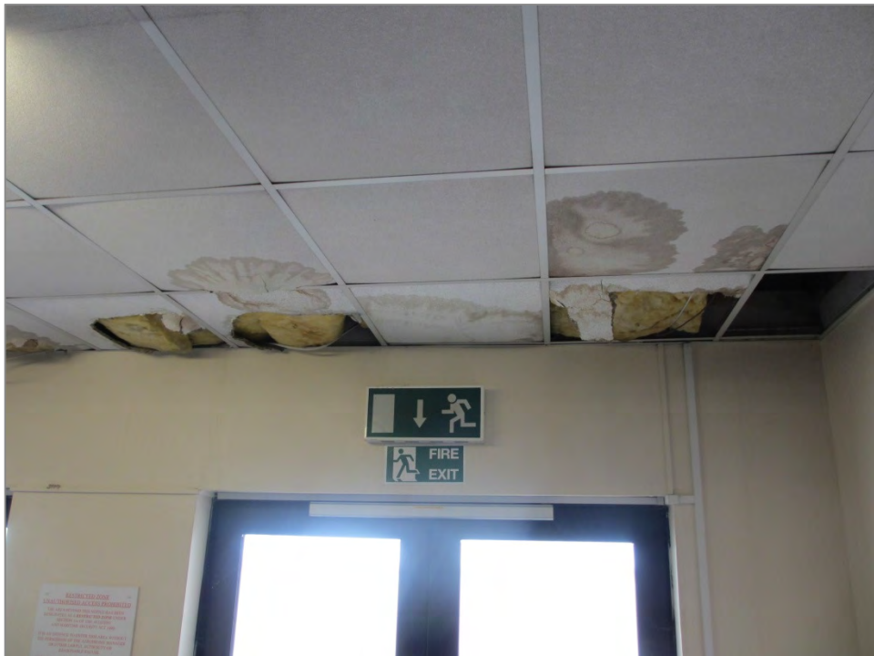
Figure 2: Evidence of water entering terminal building
