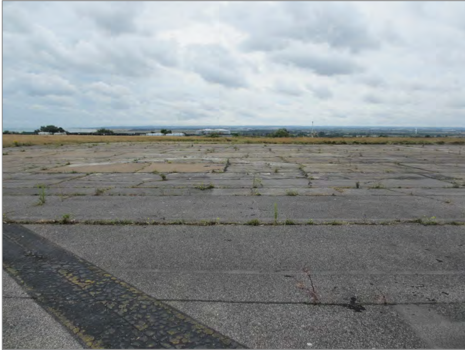
Figure 10: Shoulders of runway are paved. Evidence of plants establishing a presence in cracks
