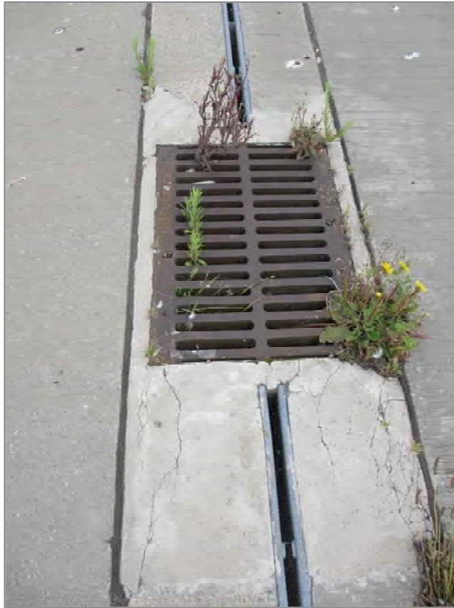
Figure 7: Apron Drainage. Some growth of plants which will need to be addressed.
