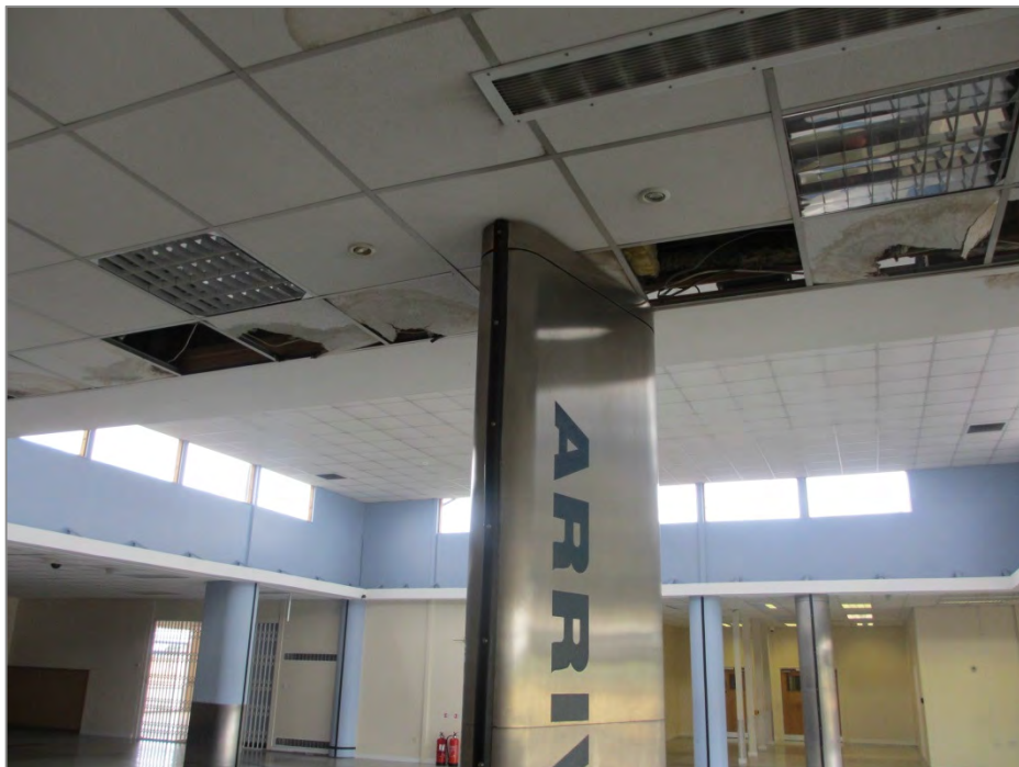
Figure 4: Evidence of water damage in main foyer.
