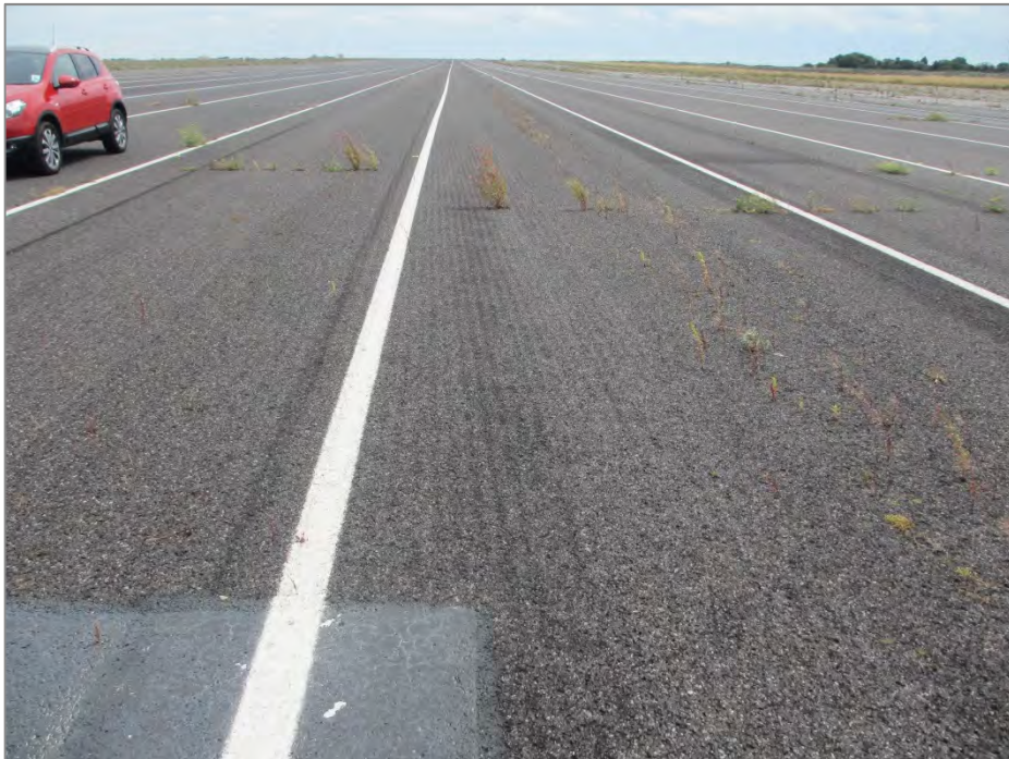
Figure 11: Runway 27 and evidence of plants establishing presence in cracks
